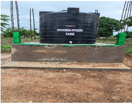
This is their new holding tank for the well water.
